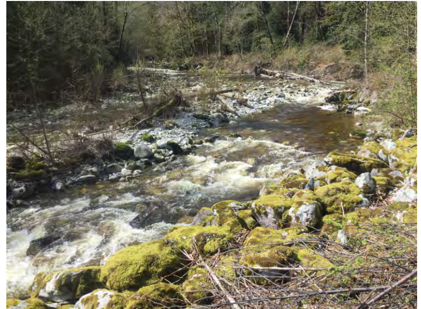
Looking upstream. Note scoured bank on right.
